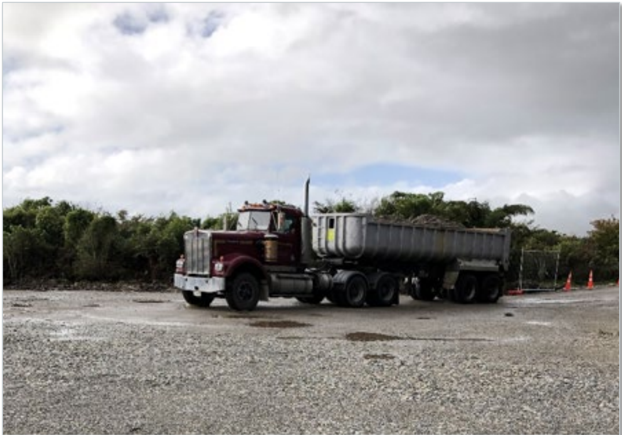
Figure 28 - Earthworks for Temporary Accommodation Service at Alma Rd (photo courtesy Pam Johnston)
